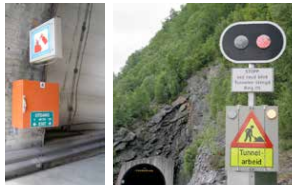
Fire extinguisher and stop signal/signs when a tunnel is closed.
