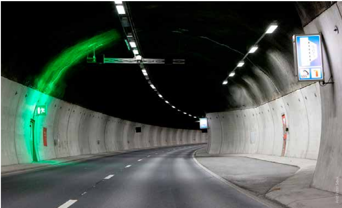
Tunnel with marked, lighted emergency exits, emergency niche and emergency telephone/fire extinguisher.
