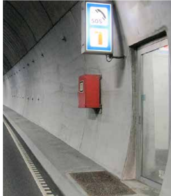
Emergency telephone and fire extinguisher in tunnels.
